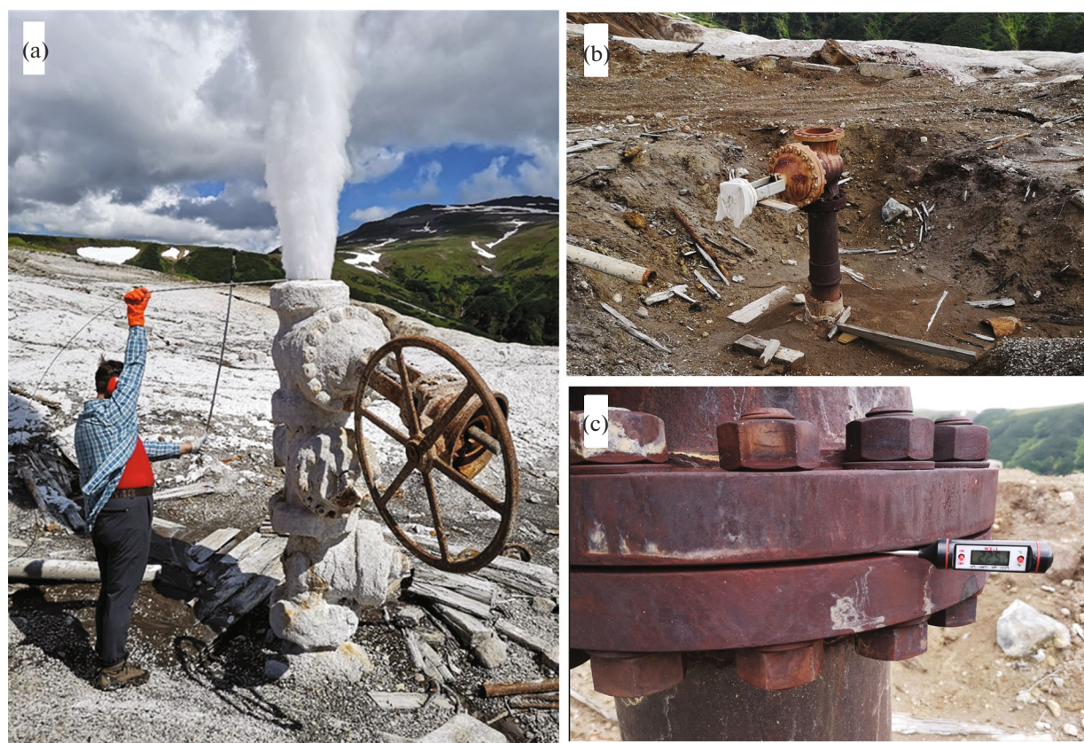
Fig. 1. The blowing well 022 in the southeastern flank of the Mutnovsky geothermal field (for the location of the well see Fig. 2), in the background is a layer of “silicate snow” (see subsection 4.4), considerable decreases in two-phase blowing wellhead temperature (down to 85°C at atmospheric pressure) were observed there since 2019, the photograph was made in 2020 (a); (b) well 022 after closing the control valve in 2022; (c) head of well 022 with measured temperature 225°C.
